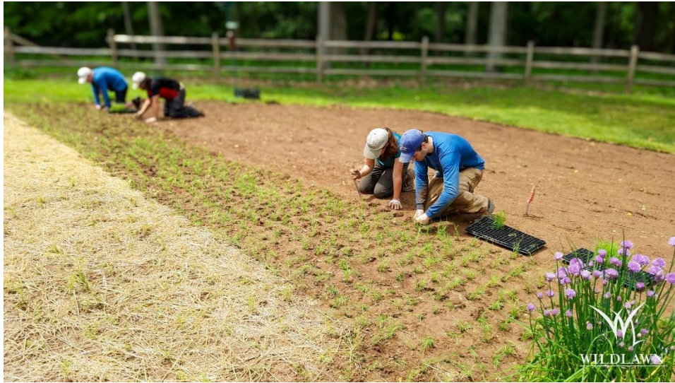
Figure 46 - Yes, meadows can be installed using tightly spaced plugs, as shown in this image. This technique is best for meadows under an eighth of an acre
